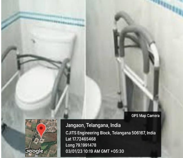
Fig 7: Western Toilet for Physically-Challenged
